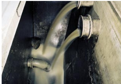
Saugraum, Abwasserpumpwerk | Suction room, Sewage pump station
