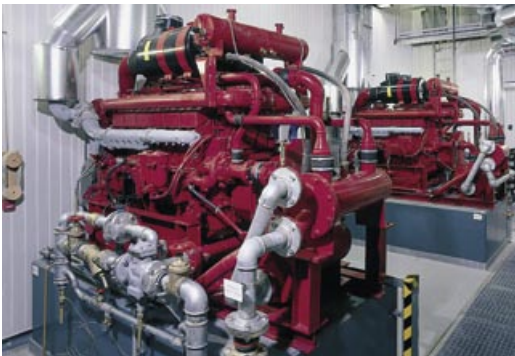
Maschinensatz, Abwasserpumpwerk | Machine set, Sewage pump station
