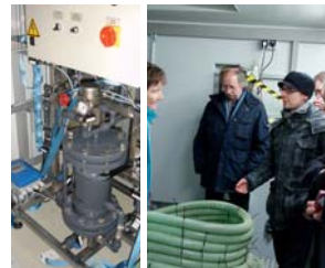
Pilotanlage Tegeler See Pilot plant at Lake Tegel
