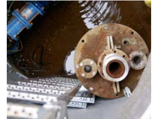
Verockerte Steigleitung Brunnen Clogged pipe (at drinking water well)
